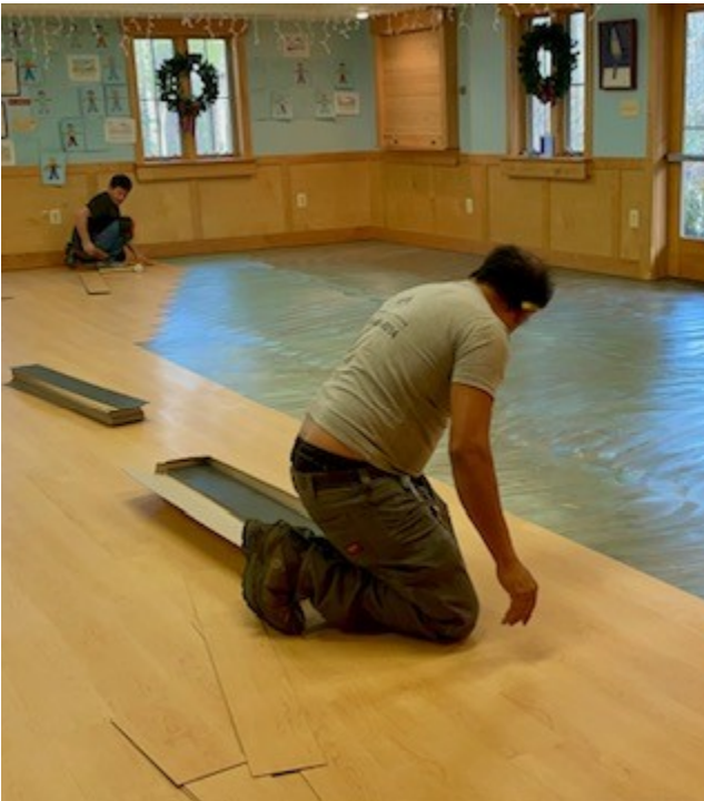
Below: New composite flooring being laid in the Richardson Room after the flooding late last year, December 12 th , 2024.
